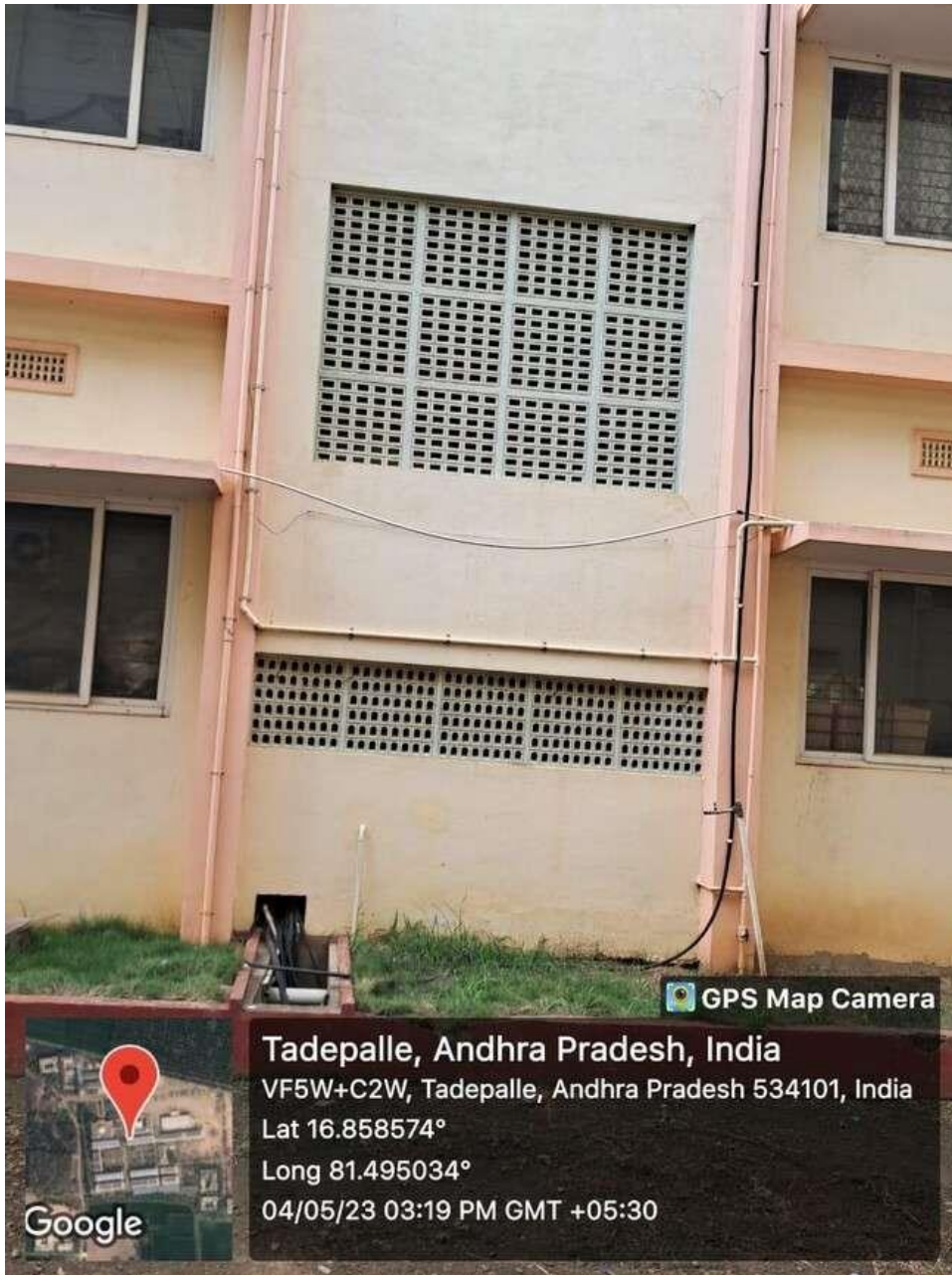
RO water distribution pipes at ECE block
