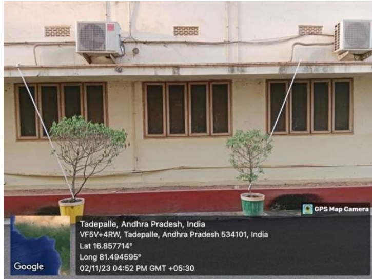
AC waste water supplied to plant
