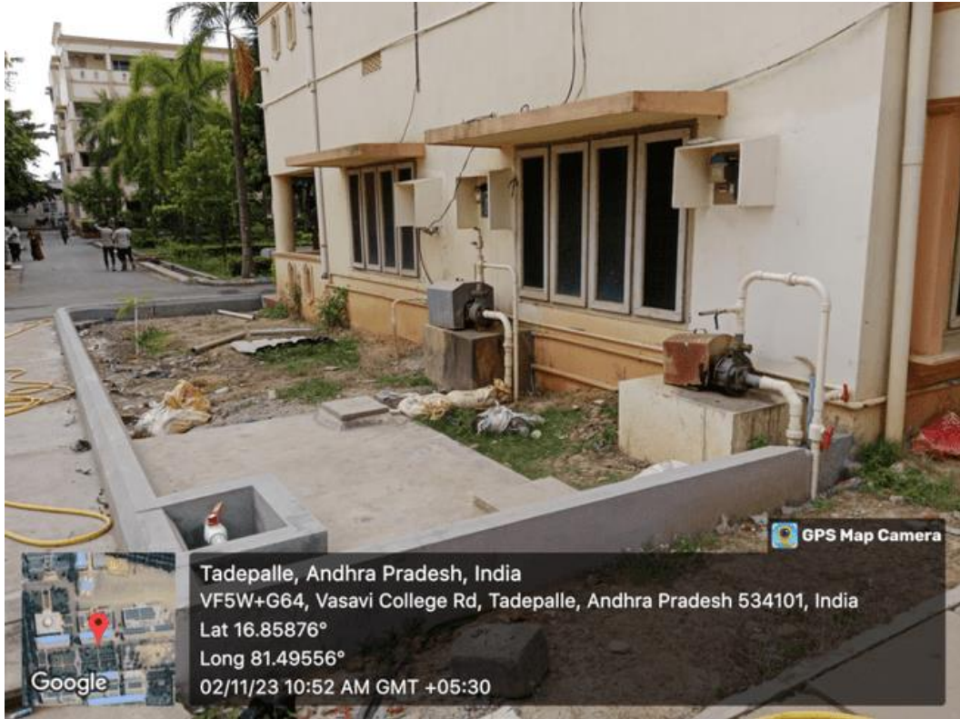
Sump with motor 3HP motor (2 numbers) are used to supply (Bore water) Auditor block And BSH block wash areas.
