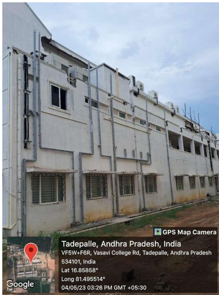
Water distribution pipes in Auditorium block
