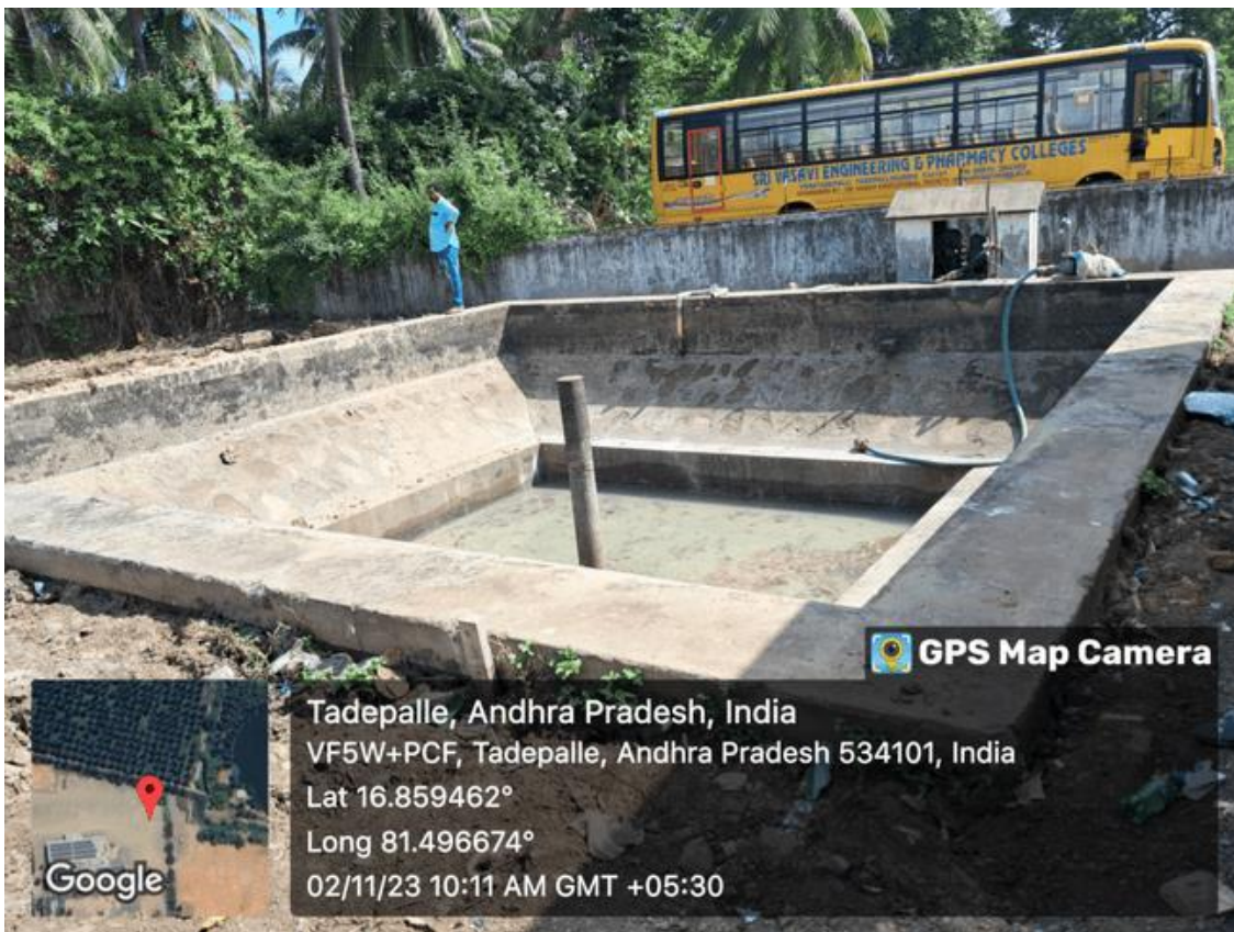
Water tank with 50000 litres capacity
